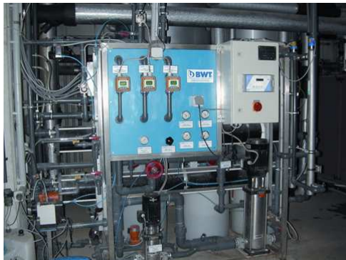
Switchboard for sewage Water Treatment and UV Radiation
